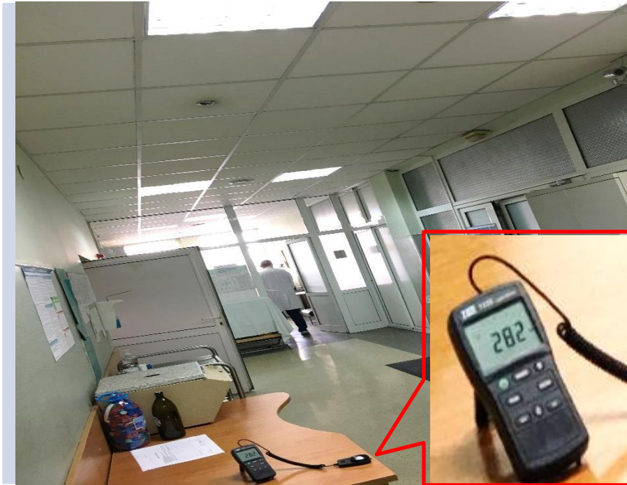
Before (T8 Lighting)
